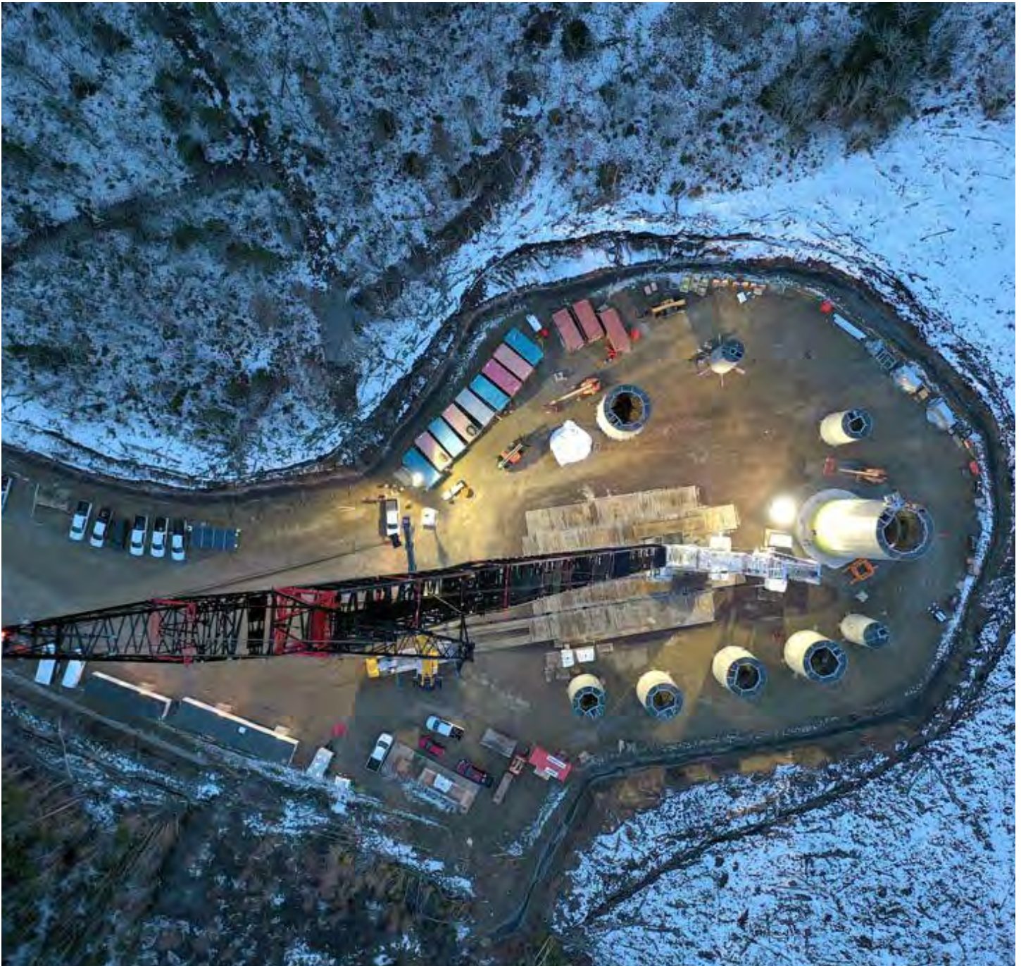
Aerial view of Oinpegitjoig (Richibucto) Project in construction, New Brunswick (Natural Forces)
